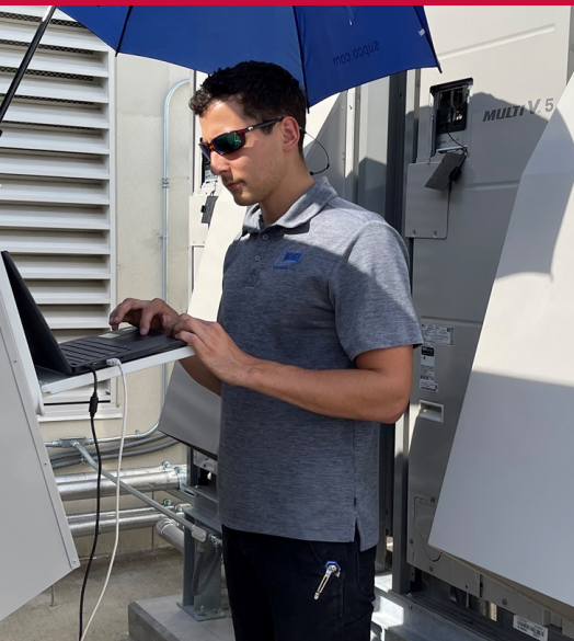
Jared Thompson, Service Manager for Encore Mechanical LLC, shown providing analysis of an HVAC system.
